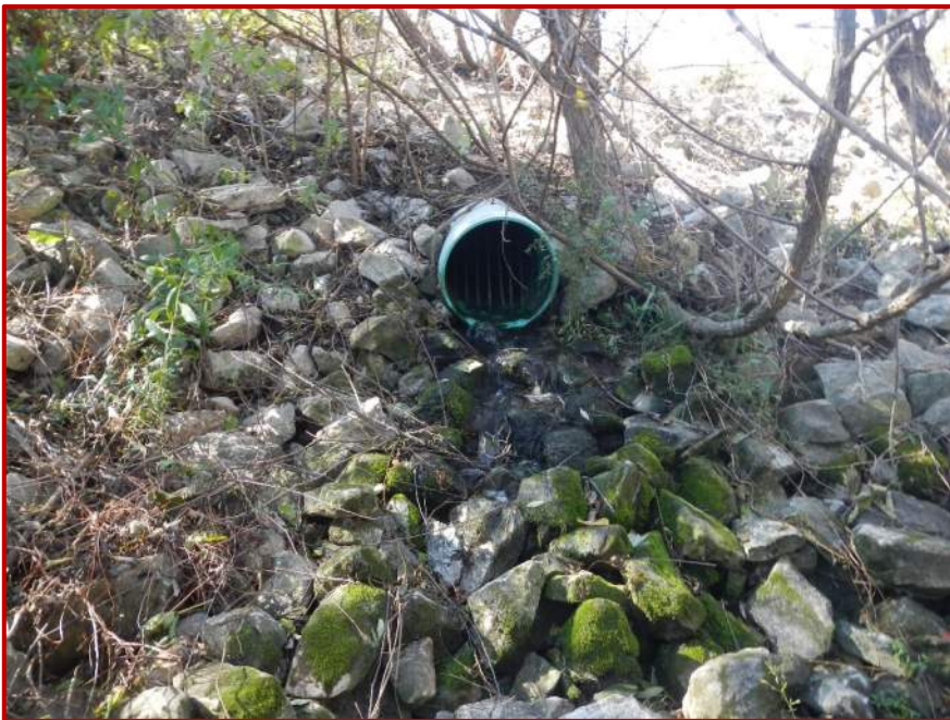
Photo 12. Looking west at the Kate Lee tile outlet which drains into School Branch within Investigated Area 2.
