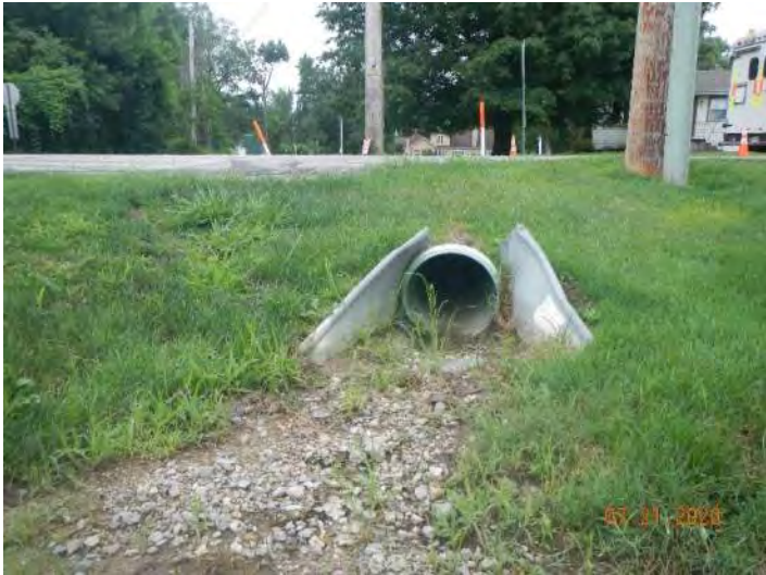
Photo 3. Looking south at a culvert located at the 5 th Street/CR 1100 N Intersection from the western boundary of the investigated area.
